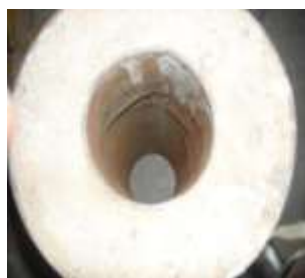
Fig. 1 Inner tube failure
